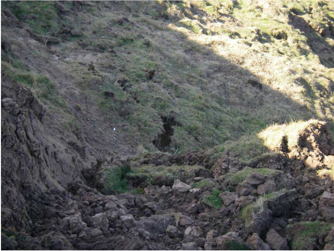
Plate 51. Site view of tension cracks in slumped glacial tills at Filey Brigg.
