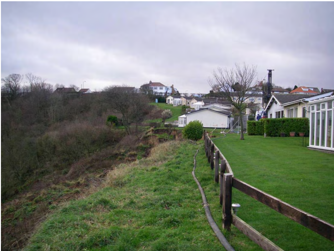
Plate 32. Site view looking south west along regressing crest showing recent failure.
