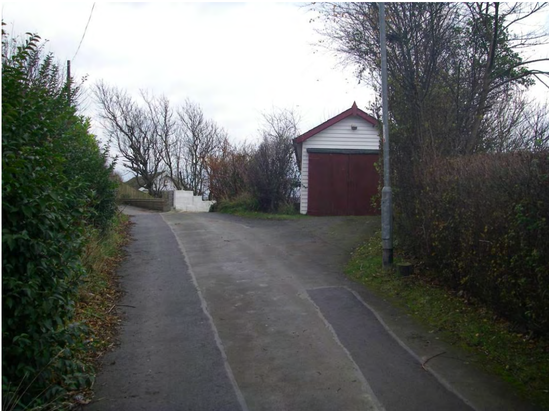
Plate 56. Site view of leaning timber garage at No. 5 Flat Cliffs, seaward of coastal slopes.
