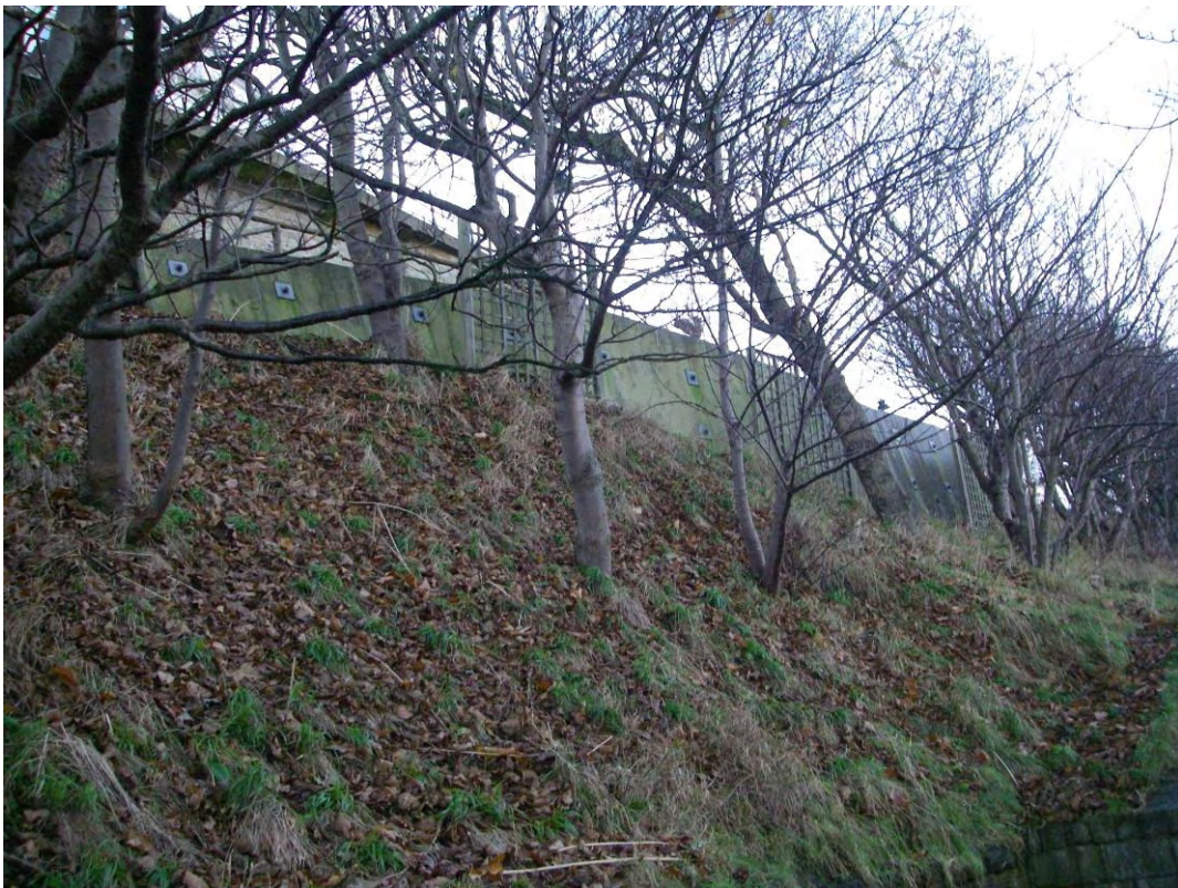
Plate 30. Site view of slope crest retaining walls at Prince of Wales Cliff.
