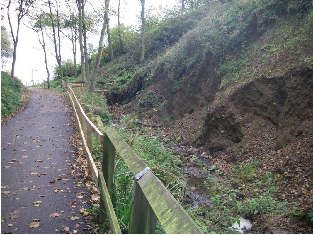
Plate 47. Site view of slope failures towards the base of Martin's Ravine.
