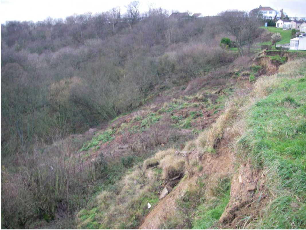
Plate 33. Site view looking south west at slope debris flow.
