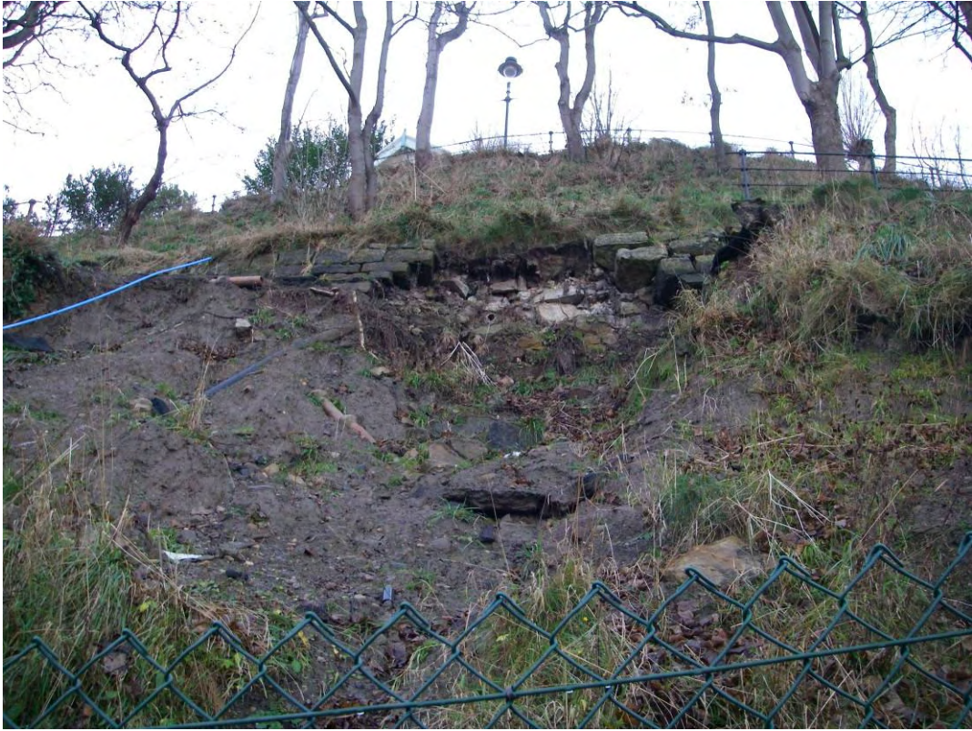
Plate 27. Site view of retaining wall and slope failure behind The Spa on Spa Cliff.
